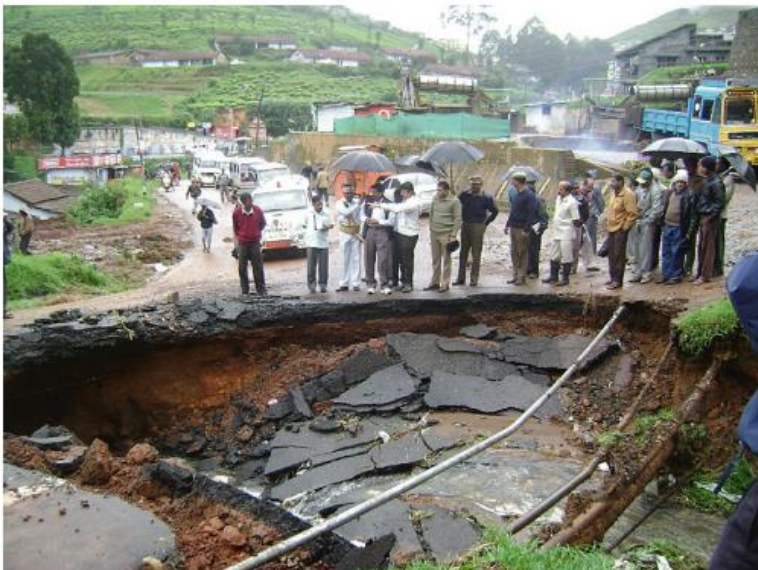
Figure 3: Severely damaged road and communication network at Ooty
